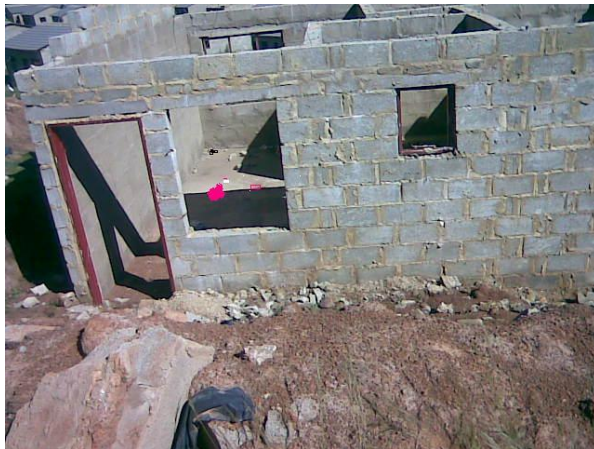
RDP Houses Mbeki, stolen window stolen window
